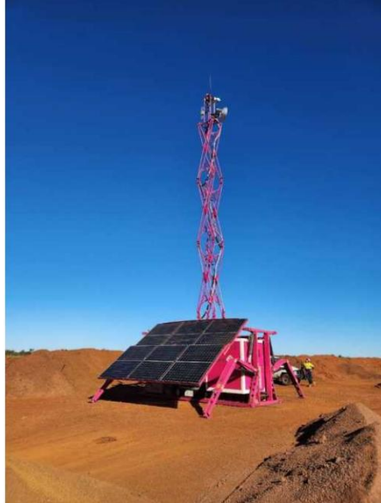
Figure 1: Nexus 16 Communication Tower deployed in the Pilbara region, Australia.
